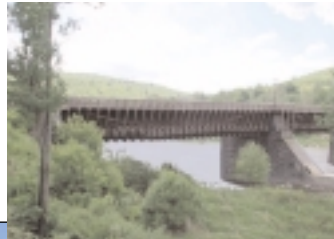
The National Park Service has issued a Special Use permit to the DVAA for the Roebling Bridge.
